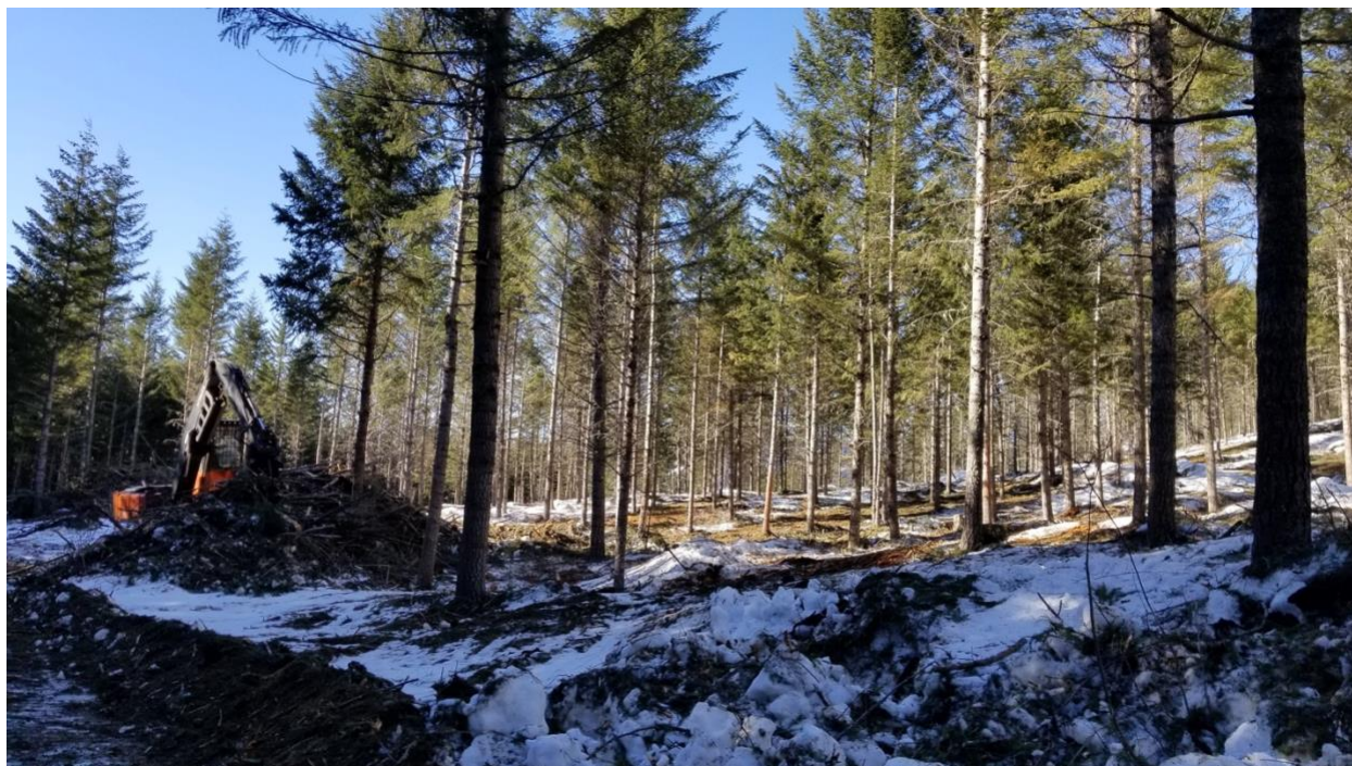
Figure 2: Phase 1 of constructing a landscape fuel break that is approximately 36 ha along Cheakamus Lake Road. Funding was provided through FESBC and the Resort Municipality of Whistler and contracted works to Lil'wat Forestry Ventures. Photo shows roadside biomass recovery: 3000m 3 was sent to the Whistler Composting Facility with the remainder chipped or burned on site.
